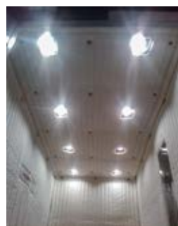
Car ceiling protection
