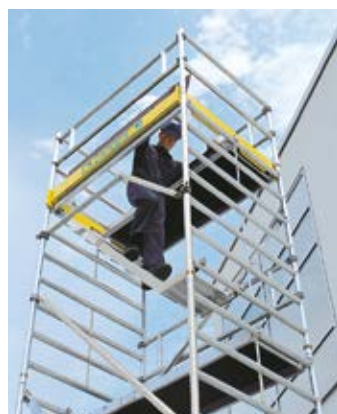
Mobile scaffolds, with supports or collapsible
